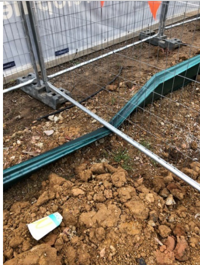
Photo 11 – Sediment fence along the east side not appropriate
