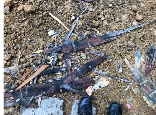
Photo 10 – Construction waste rubbish to be removed
