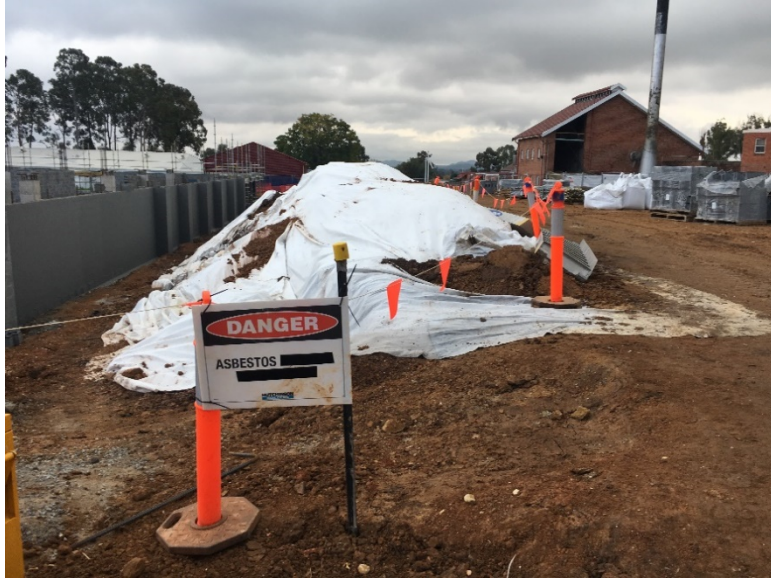
Photo 13 – Asbestos Containing Material covered and warning sign in place
