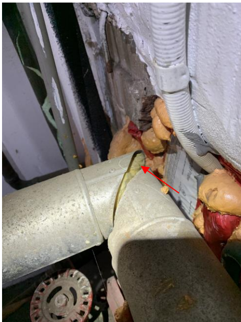
SMF encased on pipework
