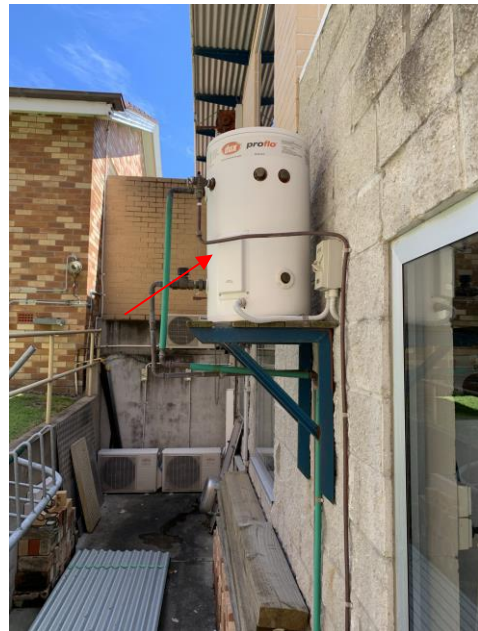
SMF: Hot water system insulation
