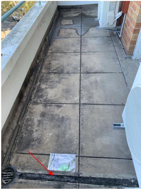
AS09 – 2: Chrysotile asbestos detected
