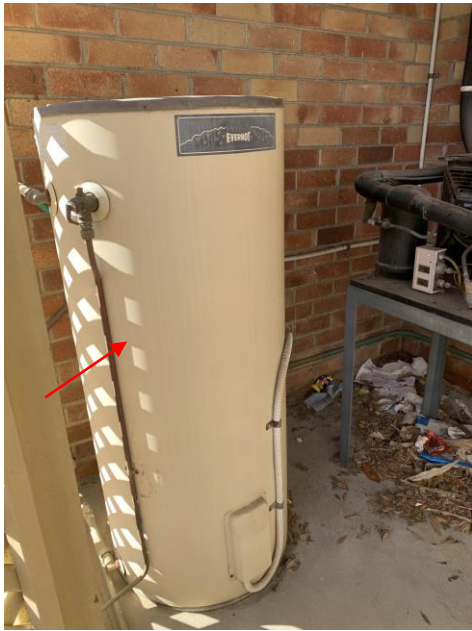
SMF: Hot water system insulation
