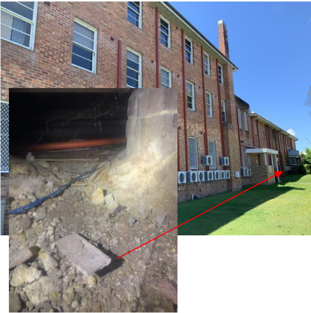
Assumed chrysotile, amosite and crocidolite debris
