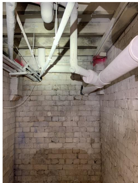
Example of subfloor surfaces following remediation in 2015. Porous and semi-porous surfaces encapsulated with white spray paint. Assumed non-friable contaminated material
