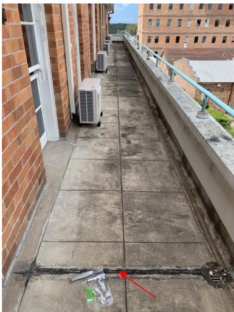
AS08 – 13: Chrysotile asbestos detected
