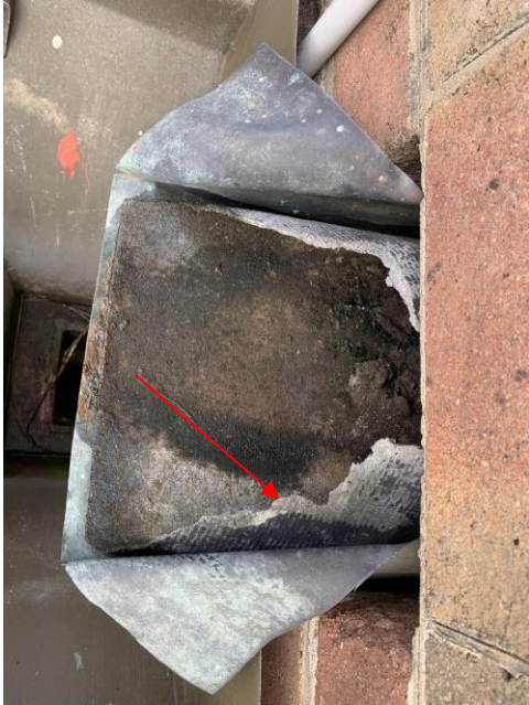
AS08 – 1: Chrysotile asbestos detected
