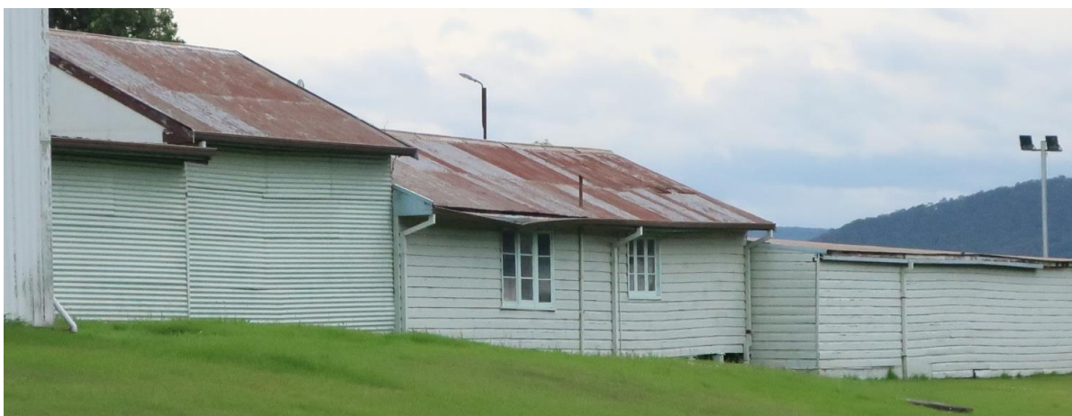
Photo 3.18 The north-western side of the shed that are Building15. The timber windows have a 1930s character. They would be demolished.
