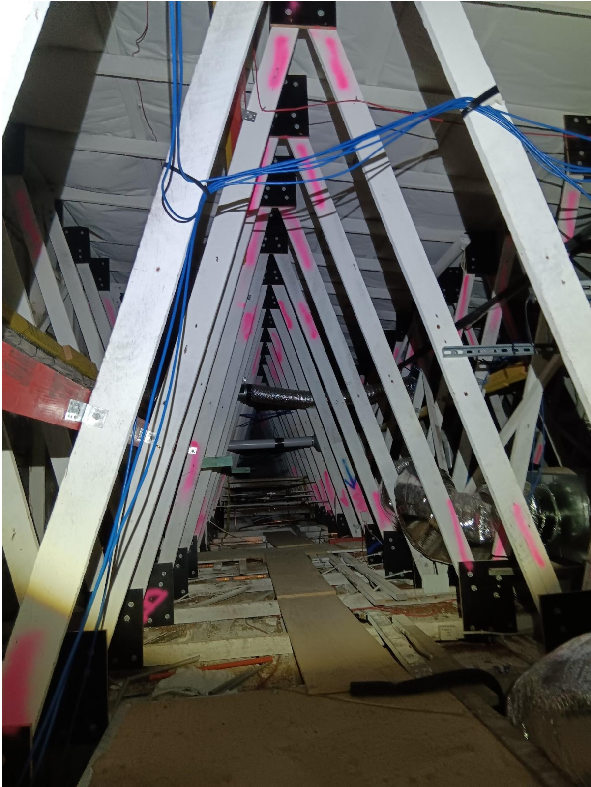
Appendix D. Photos taken during Microbat survey of roof spaces of buildings proposed to be removed.
