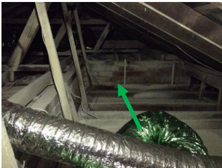
Photo No. 0112: Pharmacy Ceiling Cavity
