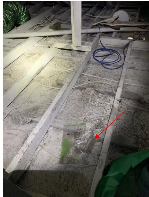
AS10 – 5: Chrysotile, Amosite and Crocidolite asbestos detected
