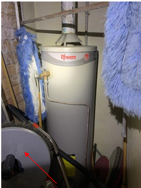
SMF – Insulation in encased hot water system
