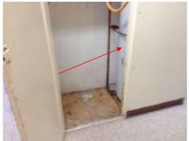
SMF: Hot water system insulation
