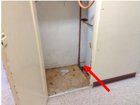
Photo No. 007: Cupboard off MN0800008
