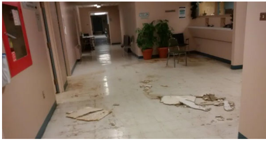
Figure 4 Even minor storm damage or flooding can stop a hospital from functioning
