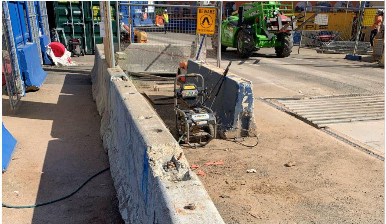
Photo 10 – High-pressure water gurney available to rinse off mud and dust from tyres
