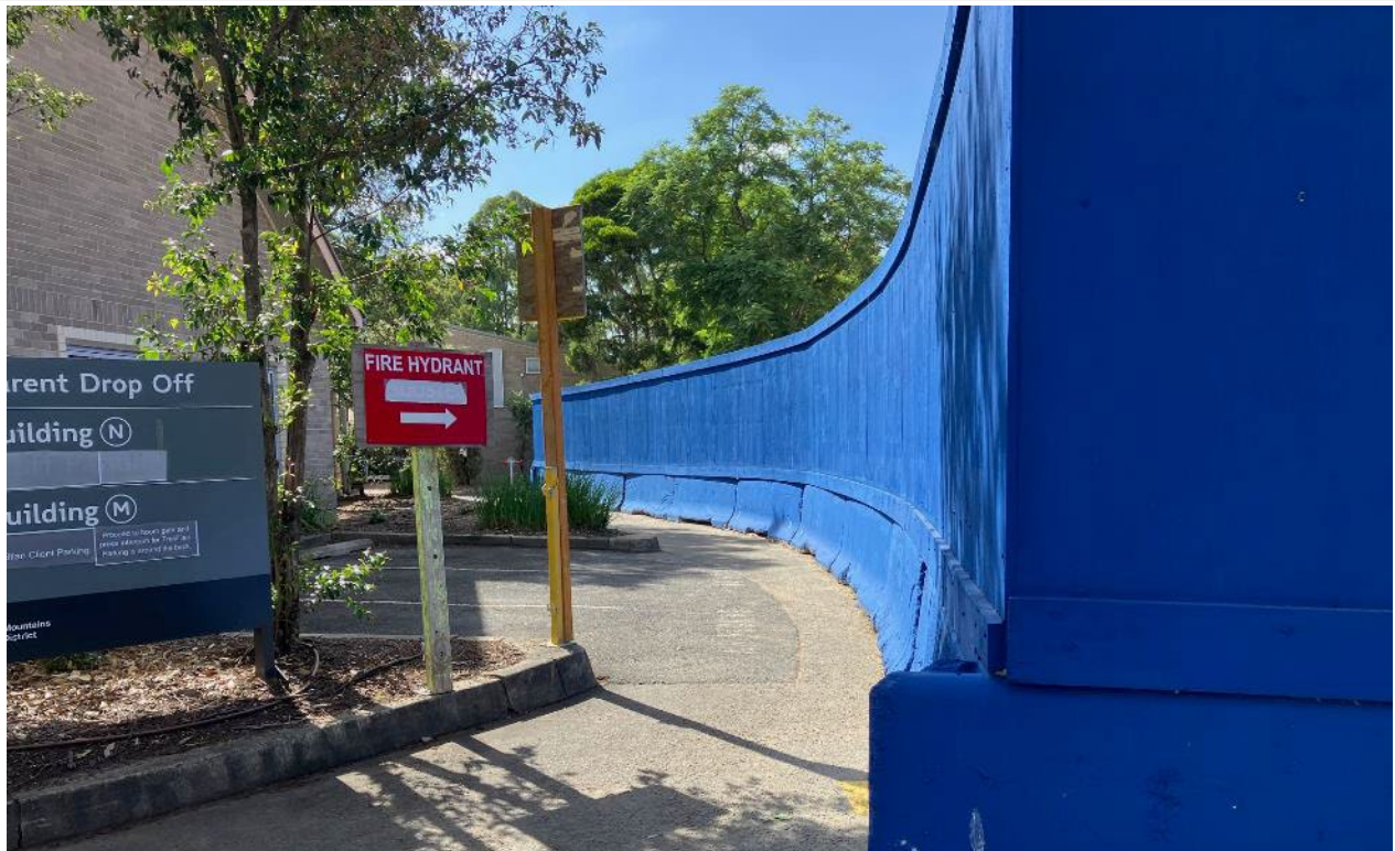
Photo 18 – Hoarding installed within the hospital grounds for stage 2 construction site to maintain pedestrian walkway.
