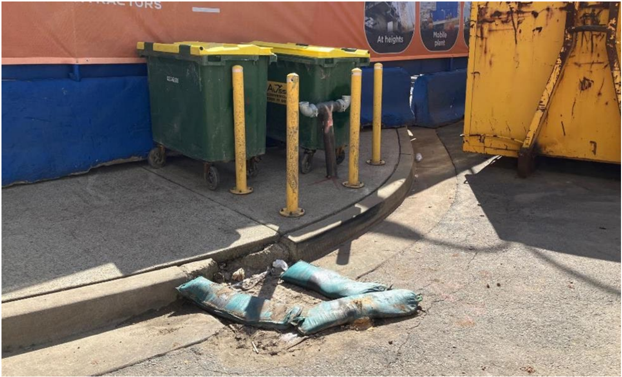
Observation 1 – Sand Bags at Barber Avenue were in poor condition
