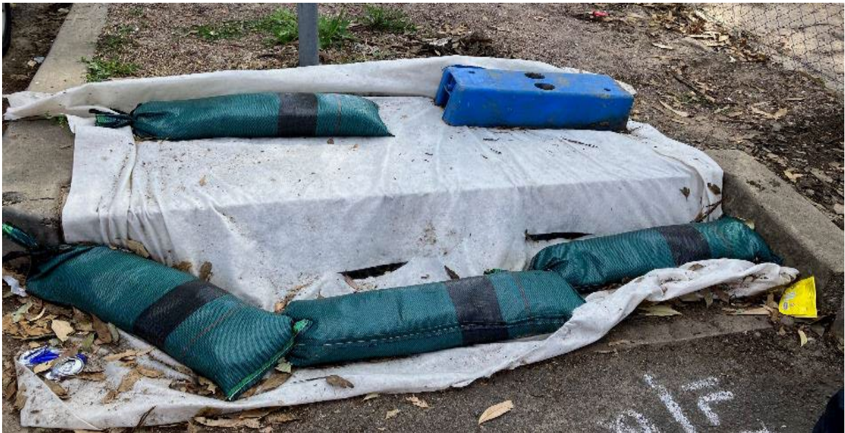
Observation 2 – Geofabric covering pit drain at Barber Avenue access was in disrepair and required replacing
