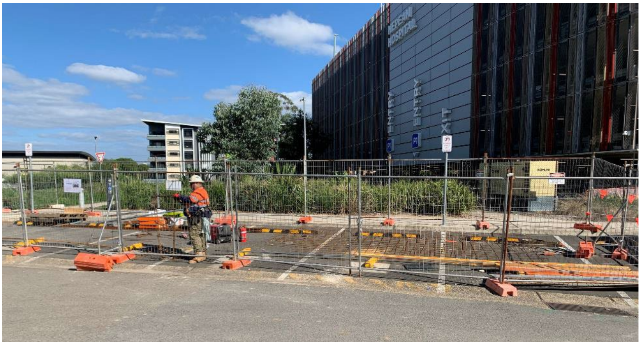
Photo 6 – Construction of Parking area next to the Loading Dock at North Block.
