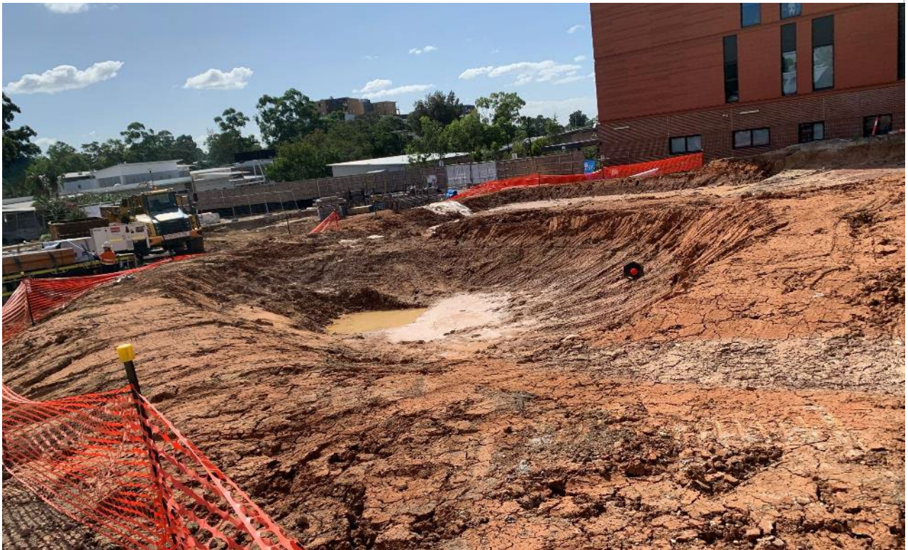
Observation 5 – No erosion and sedimentation controls or life saving devices in place for temporary sediment ponds.
