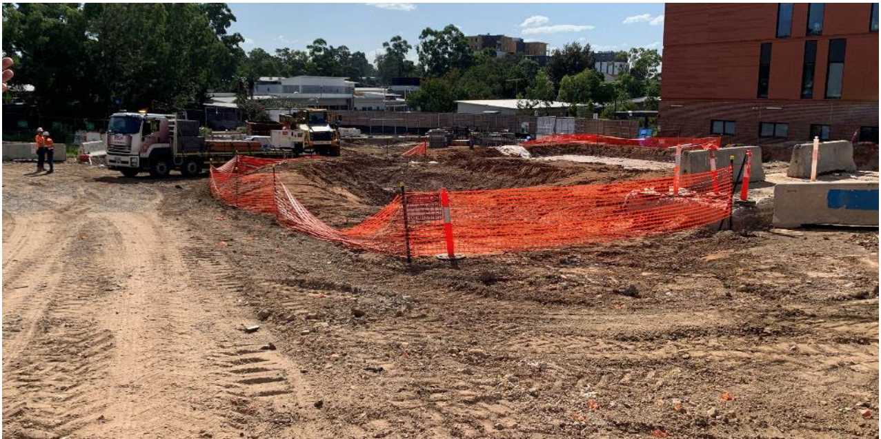
Photo 17 – Para web fencing installed at Sediment Ponds. Refer to site observations regarding controls.
