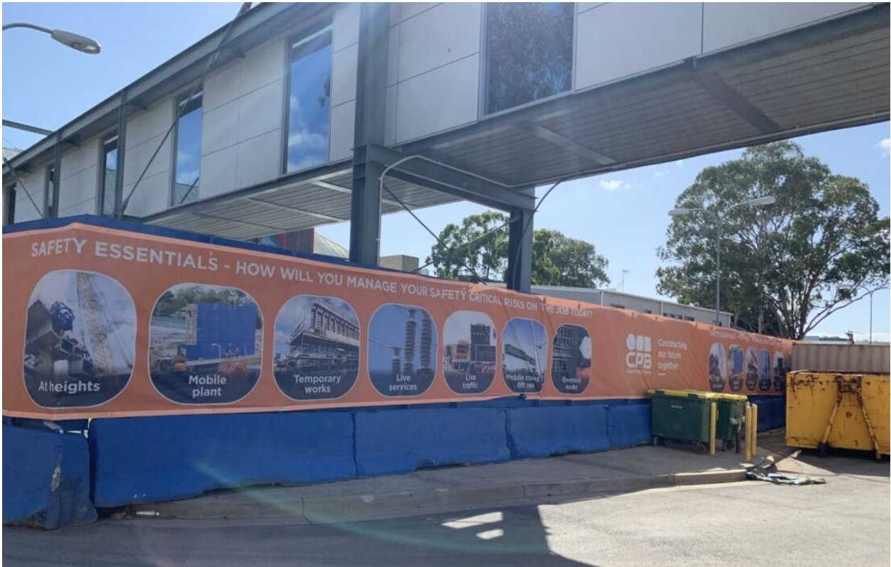
Photo 3 – Hoarding installed along the boundary of the construction site. Waste and recycling bins available.
