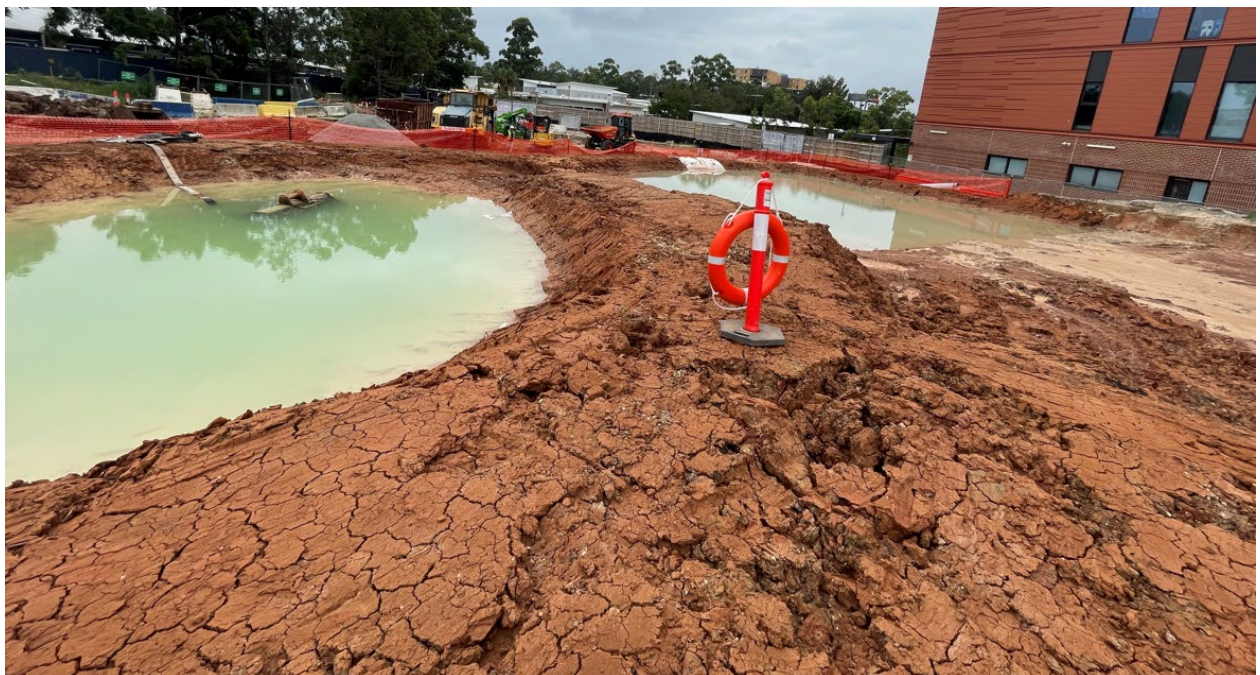
Photo provided by CPB showing lifesaving device in place. However, erosion and sediment controls did not appear adequately installed / maintained.
