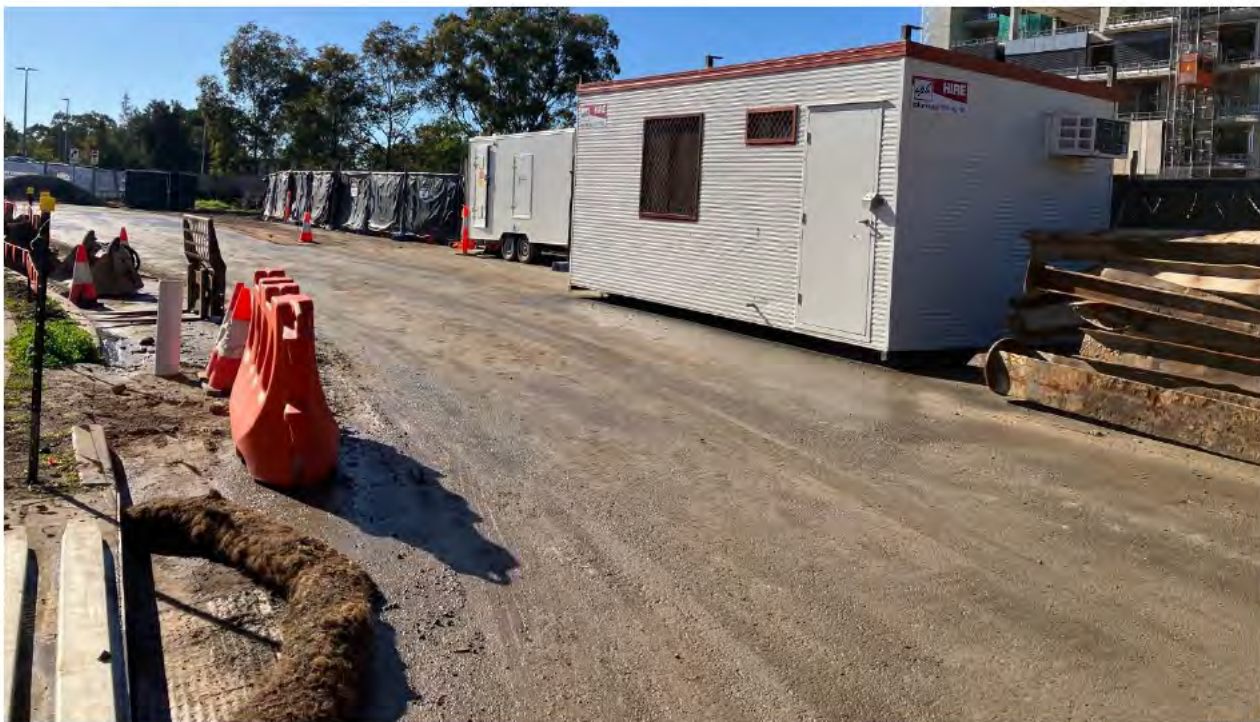
Protection of pit drain at main access road through site. Some sediment build up requiring clean up behind jersey barriers.
