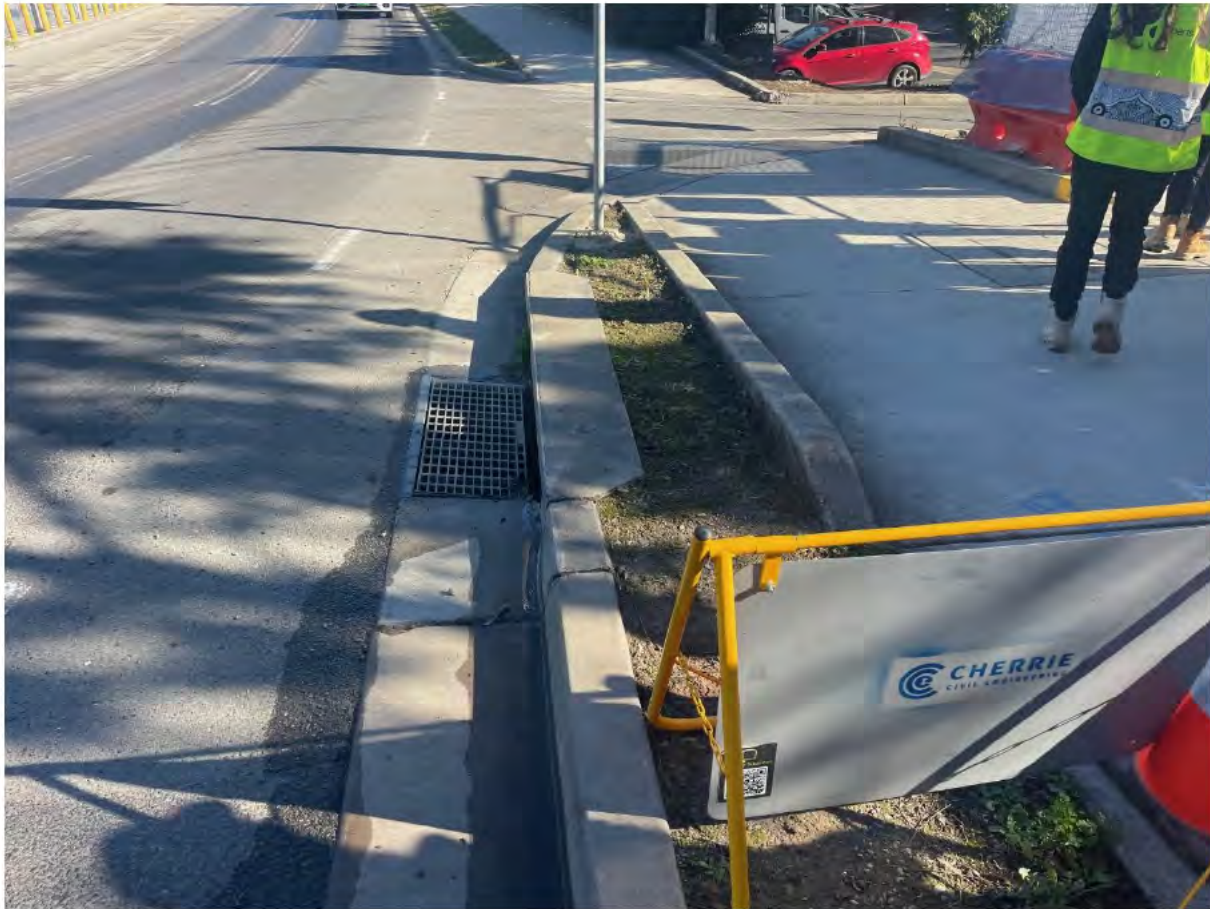
No controls in place at live drain, Redbank Road. Actioned during site inspection, refer below.
