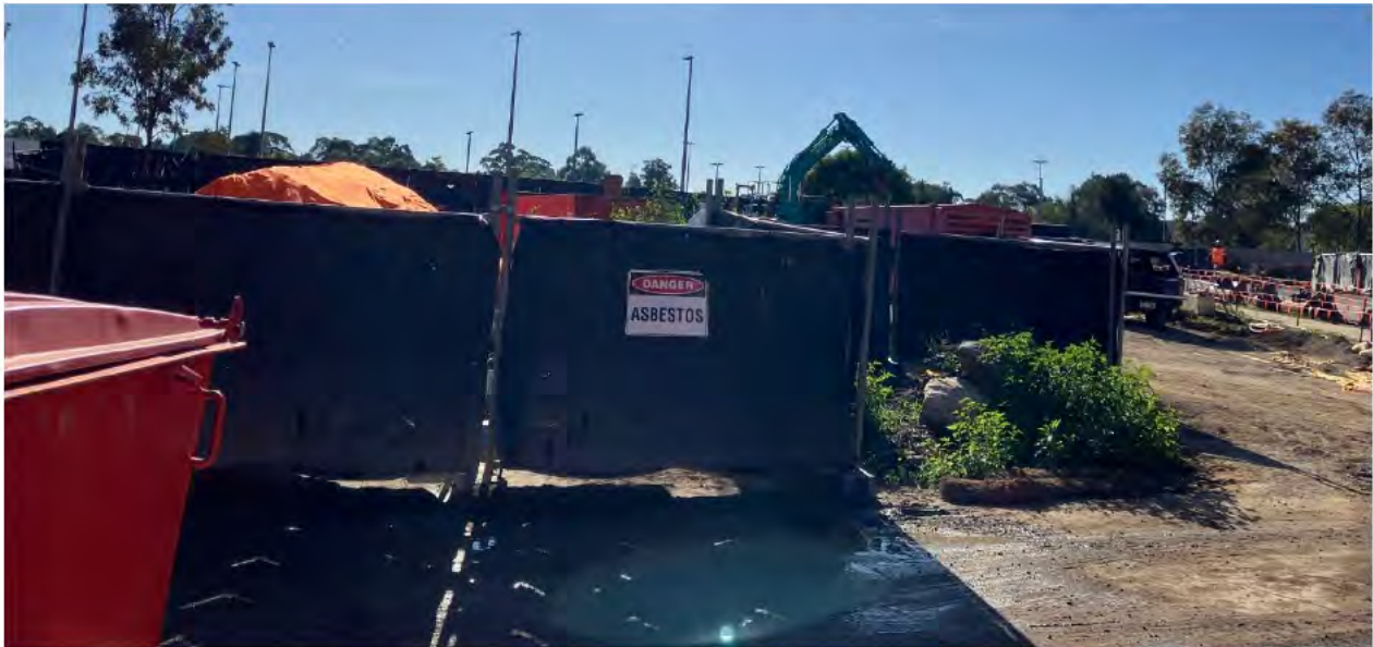
Asbestos areas are fenced with signage.
