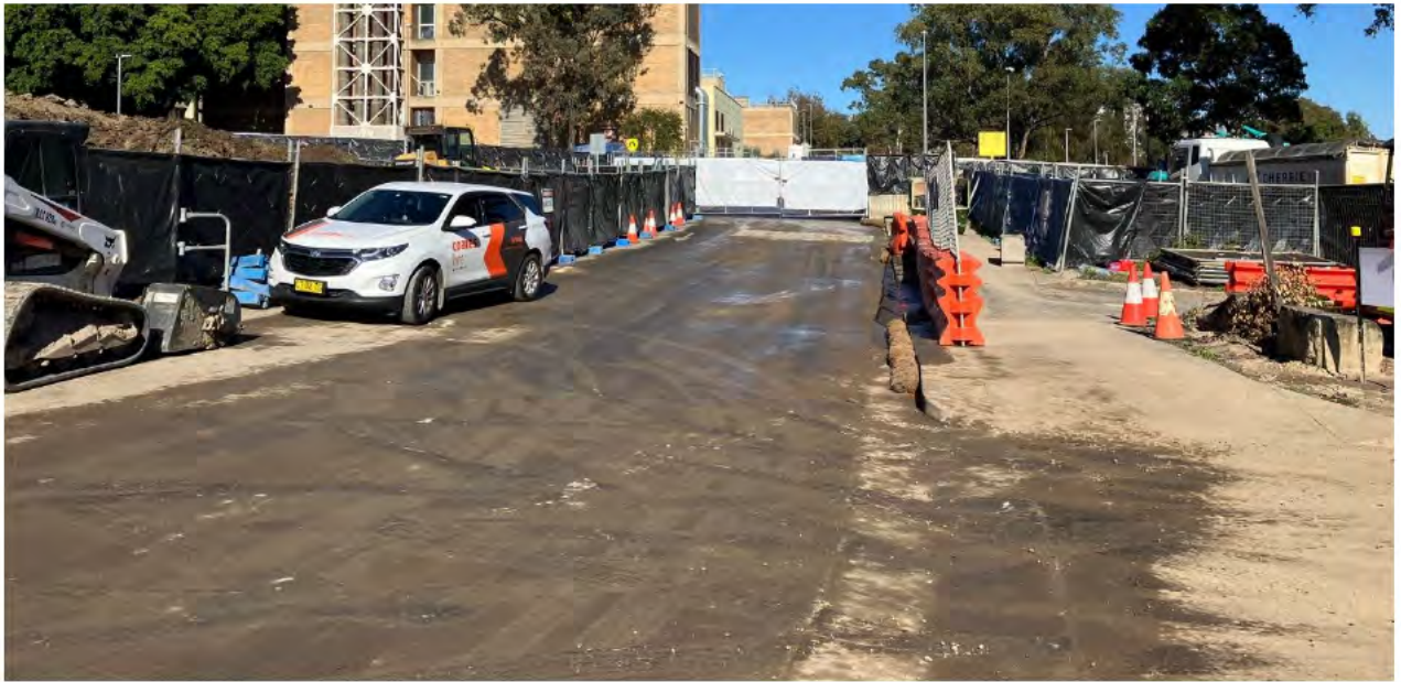
Main access road into site. Hardstand in place to reduce mud tracking and dust.
