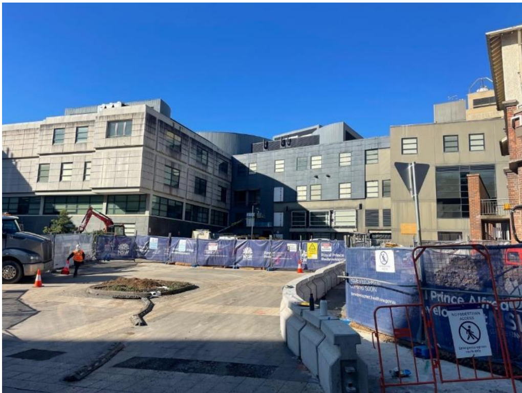
Traffic Controller in place for heavy vehicles movement at Johns Hopkins Drive.
