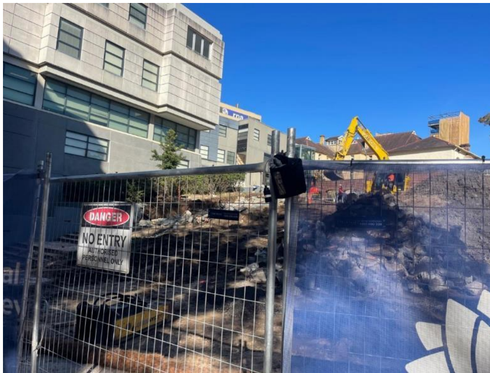
Air Quality Monitor installed on site, and monitoring results available on project website.
