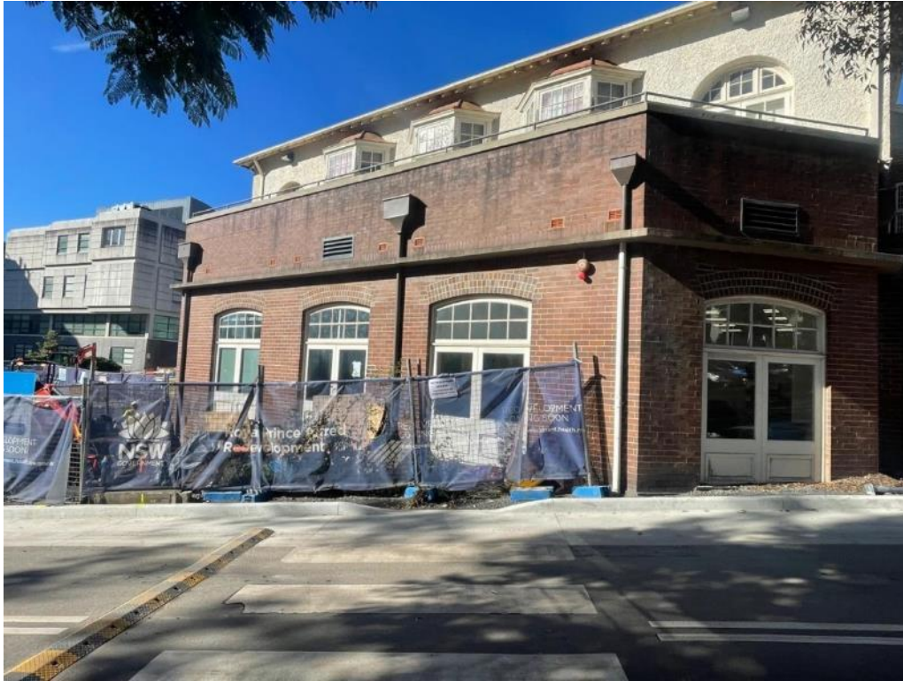
Civil earthworks in progress adjacent to the Kerry Pecker (KP) heritage building.
