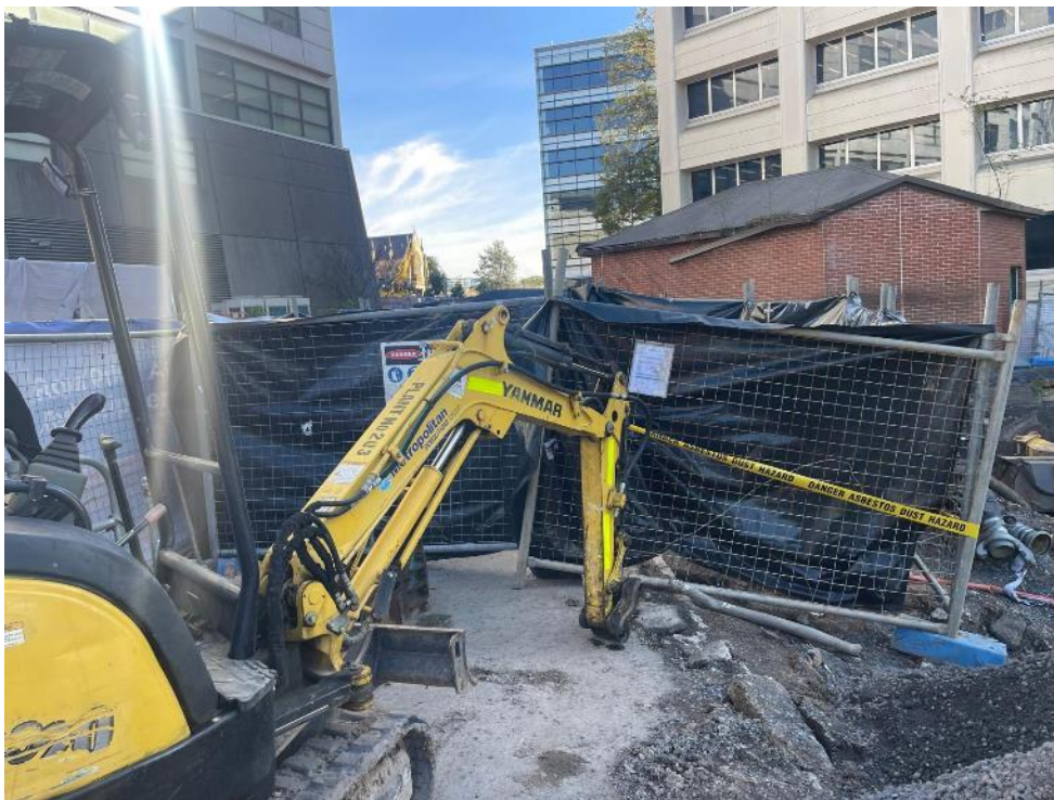
Asbestos area isolated and clearly marked for restricted access.
