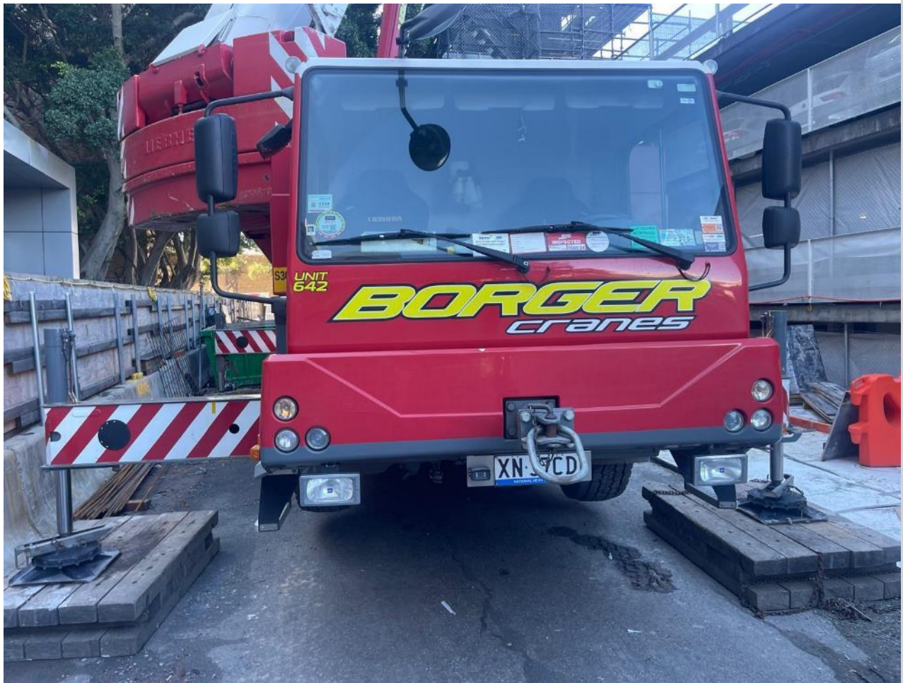
OBS-01: Borges mobile Crane located at HLS site had not turned off its engine during idling.
