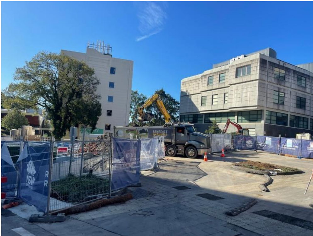
General site construction activities were in progress, with spoil being loaded into a spoil haulage truck.
