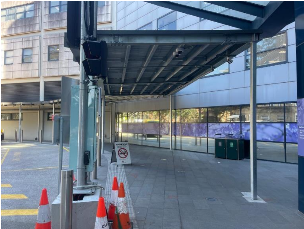
Temporary Works 1: Northern Arrival relocations, NETS and NEPT were completed and operational – OP1.
