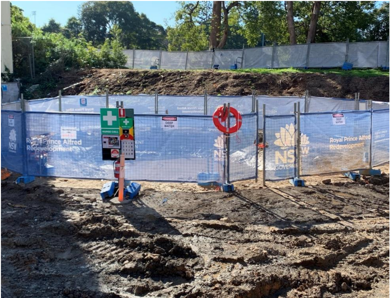
Sediment basin fenced off, and a nurse call system along with a lifesaving device in place.
