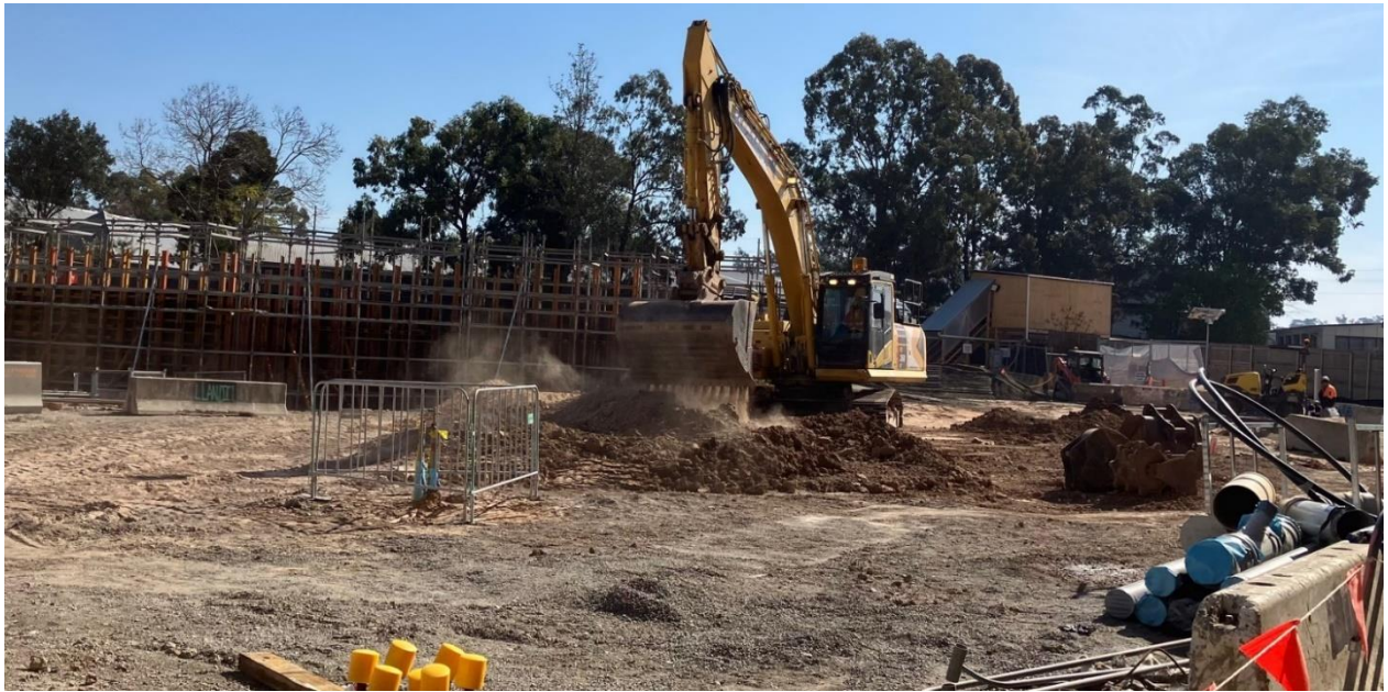
Dust observed during some site activities. Refer to NHRS2-02_OFI-06.
