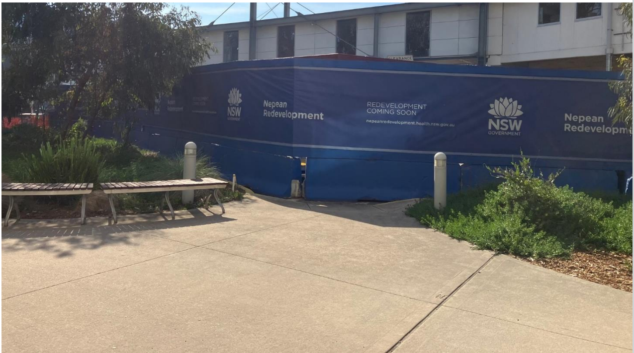
Shade cloth around site. Public areas noted to be clean and maintained.
