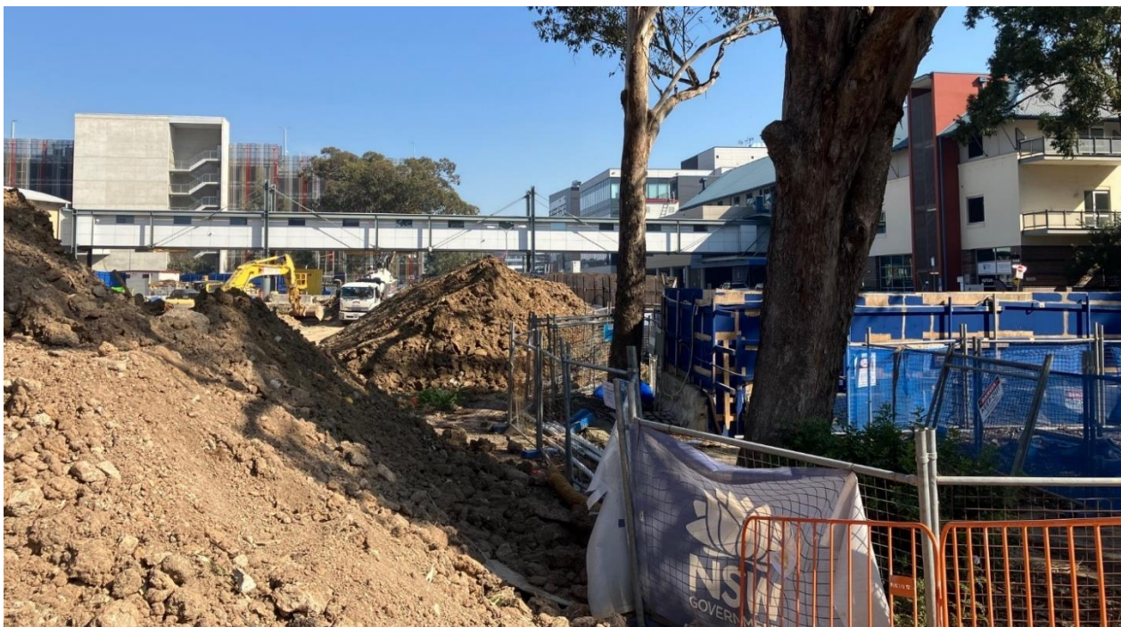
Large stockpile bordering on tree protection zone. Refer to NHRS2-02_OFI-05.
