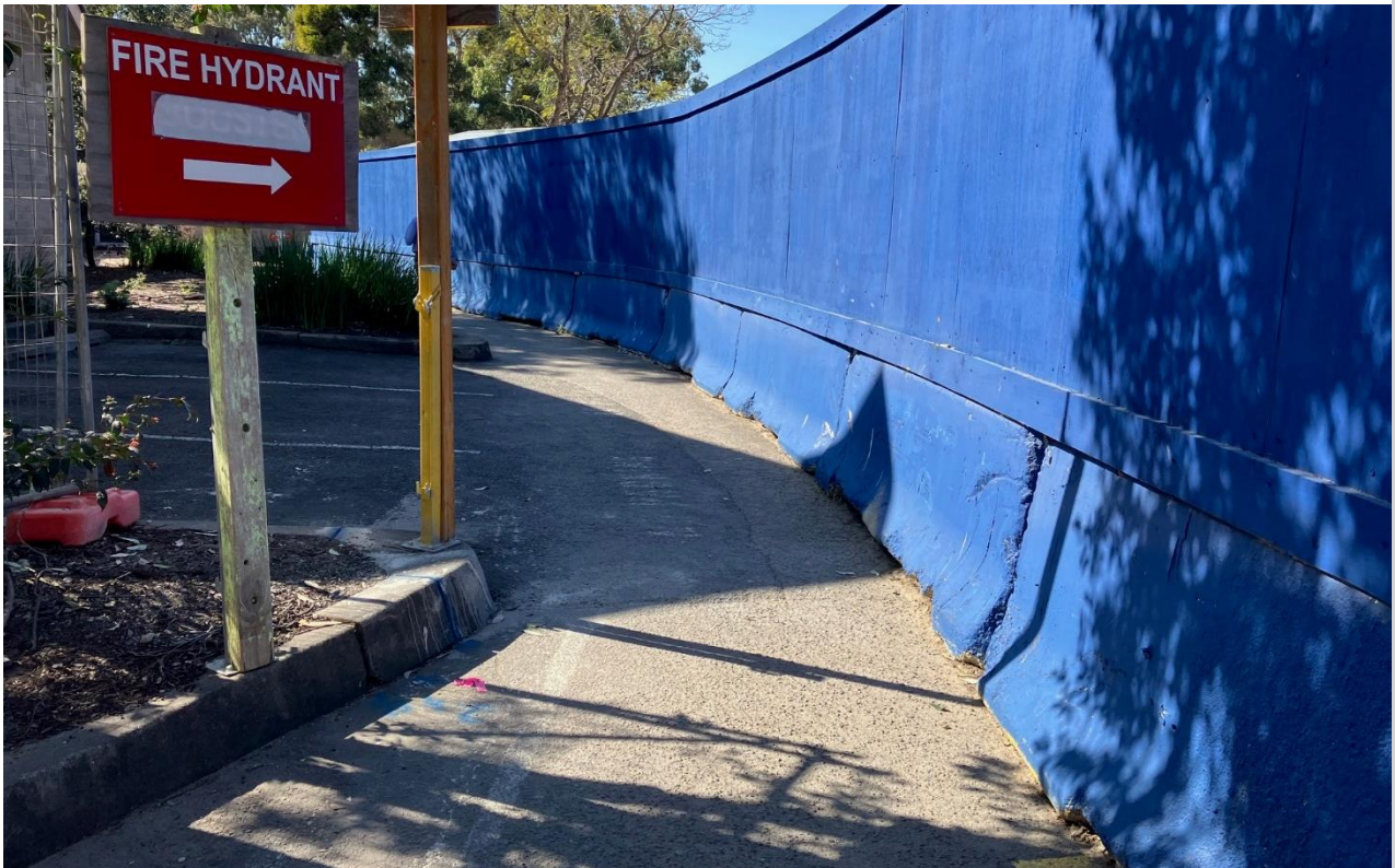
Hoarding installed at site boundary. Pedestrian access maintained and kept clean and clear.
