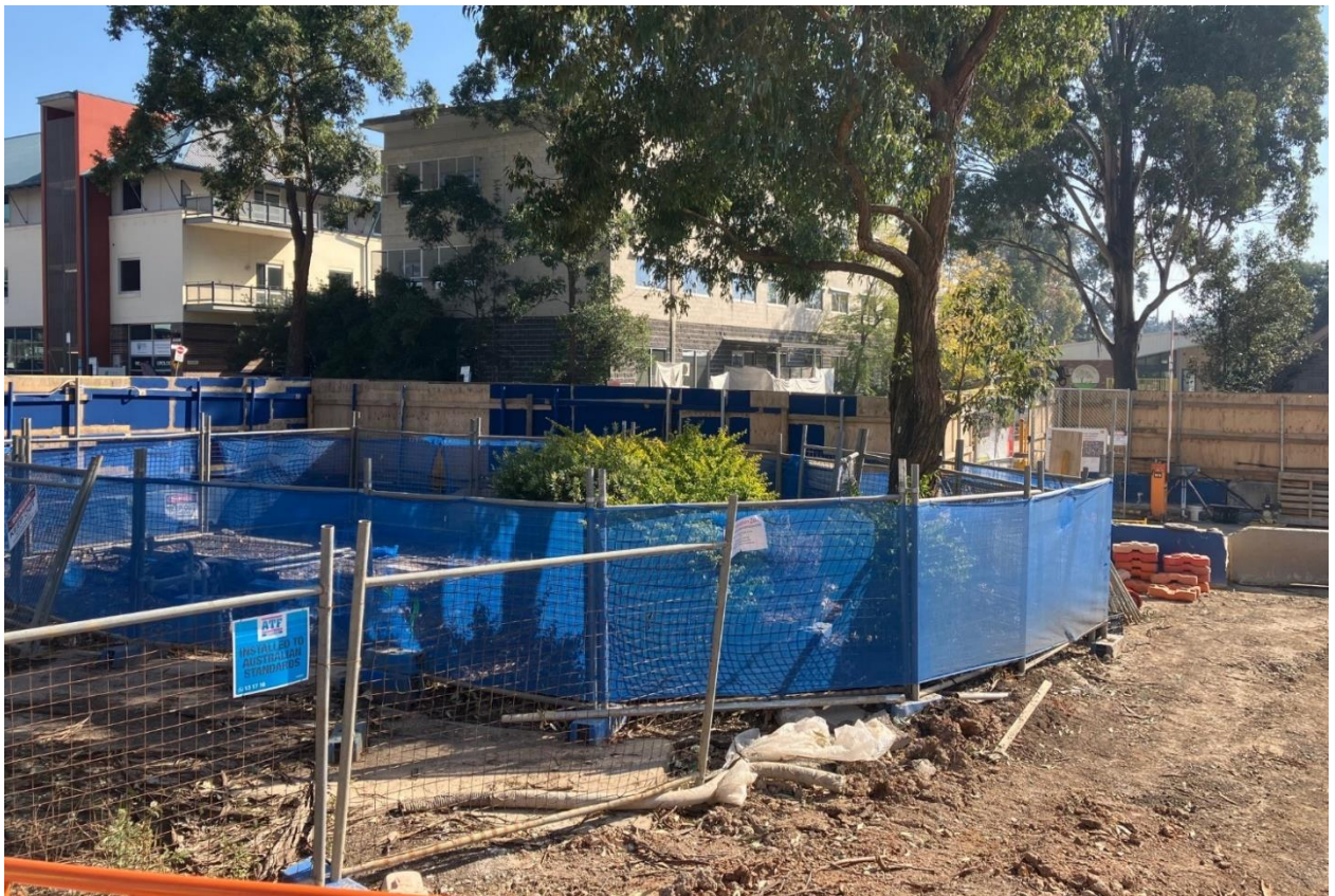
General maintenance required at tree protection areas. Refer to NHRS2-02_OFI-05.
