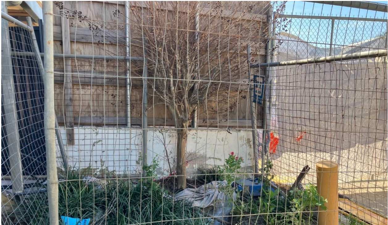
As above, clarification of fenced area as tree roots exposed and appeared be in poor condition. Refer to NHRS2-02_OFI-05.
