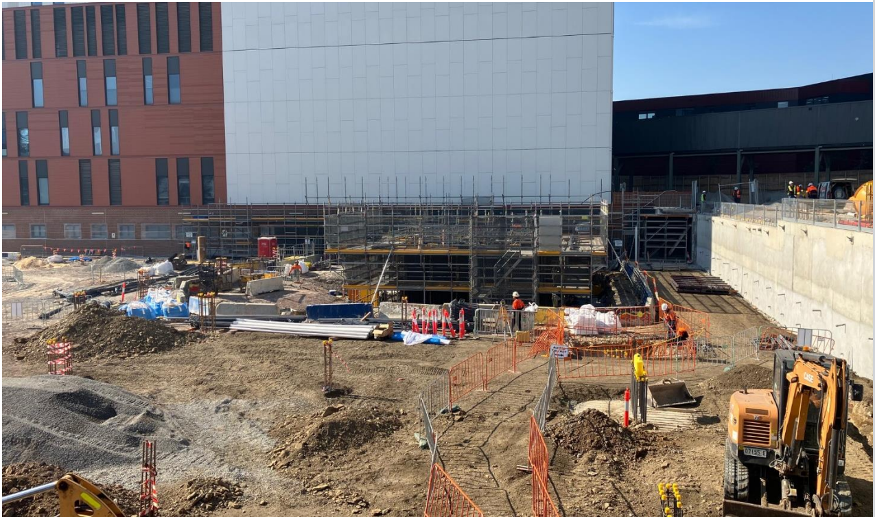
Jump form installation. Link bridge to be constructed at Stage 1 Tower A
