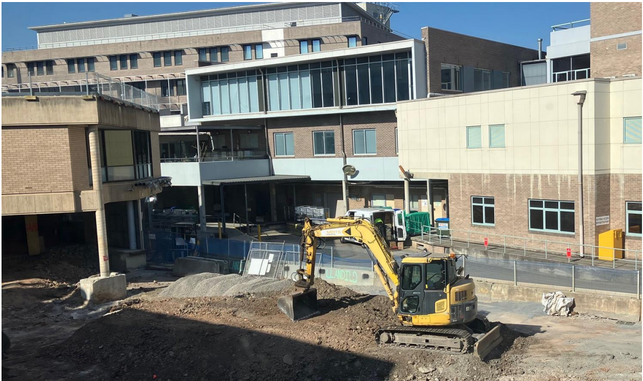
Demolition being completed in stages with loading dock area to be completed following construction of temporary loading dock.
