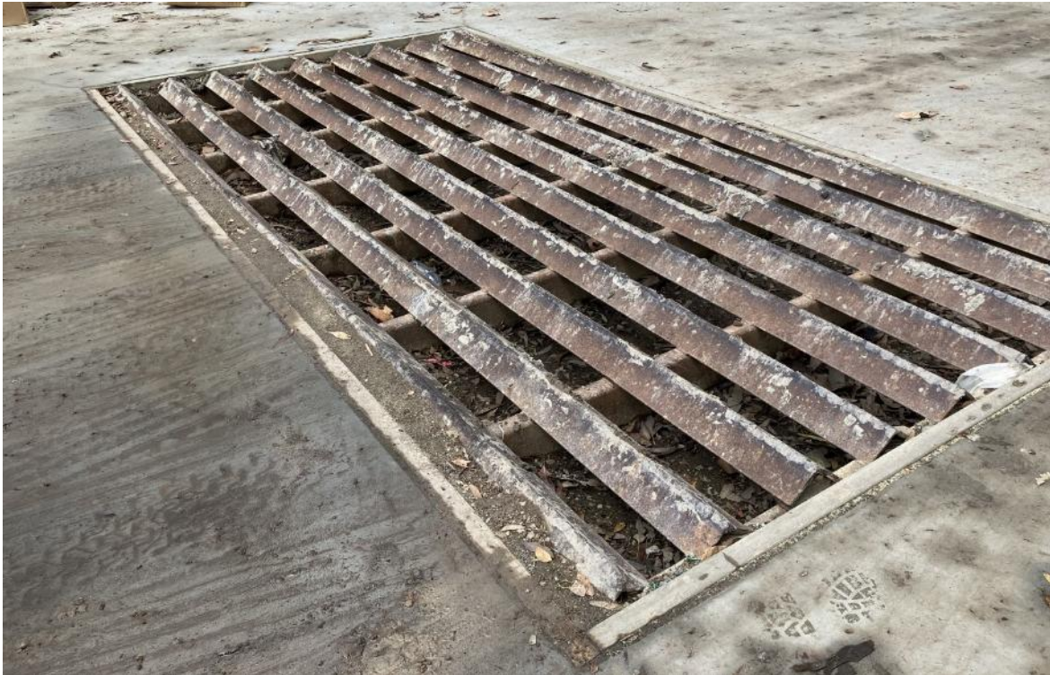
Rumble grid is in place, and the site entrance has been stabilized.
