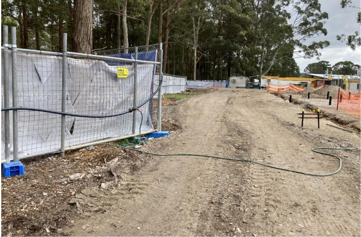
Potable hose line is available for dust suppression and vehicle cleansing.
