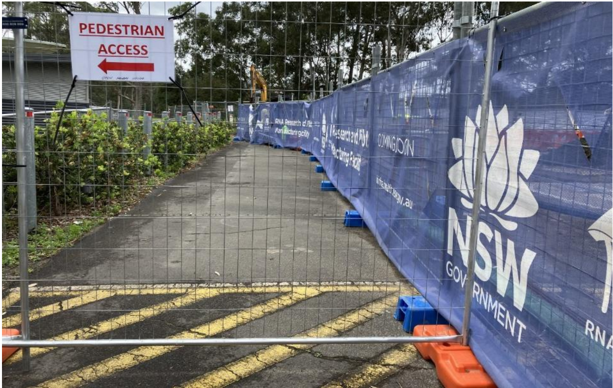
Pedestrian access signage is in place; pathway kept clean and clear.
