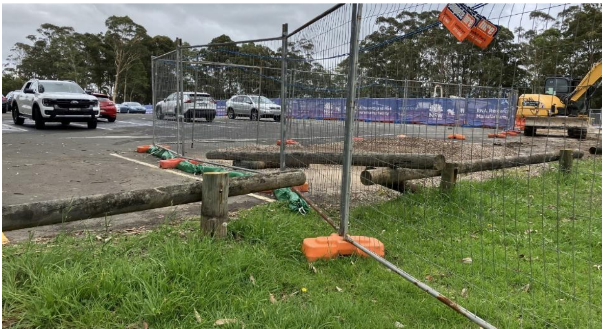
Erosion and sediment controls in place with ATF fencing adjacent to carpark.
