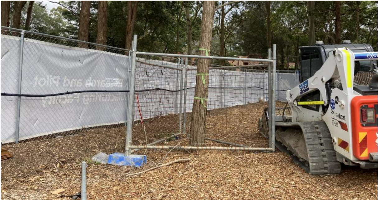
OBS-02: Tree Protection Zone sign missing.
