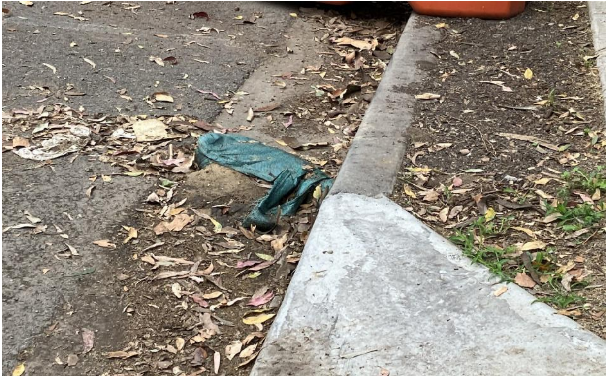
OBS-03: Sand bag at Culloden Road required replacing.
