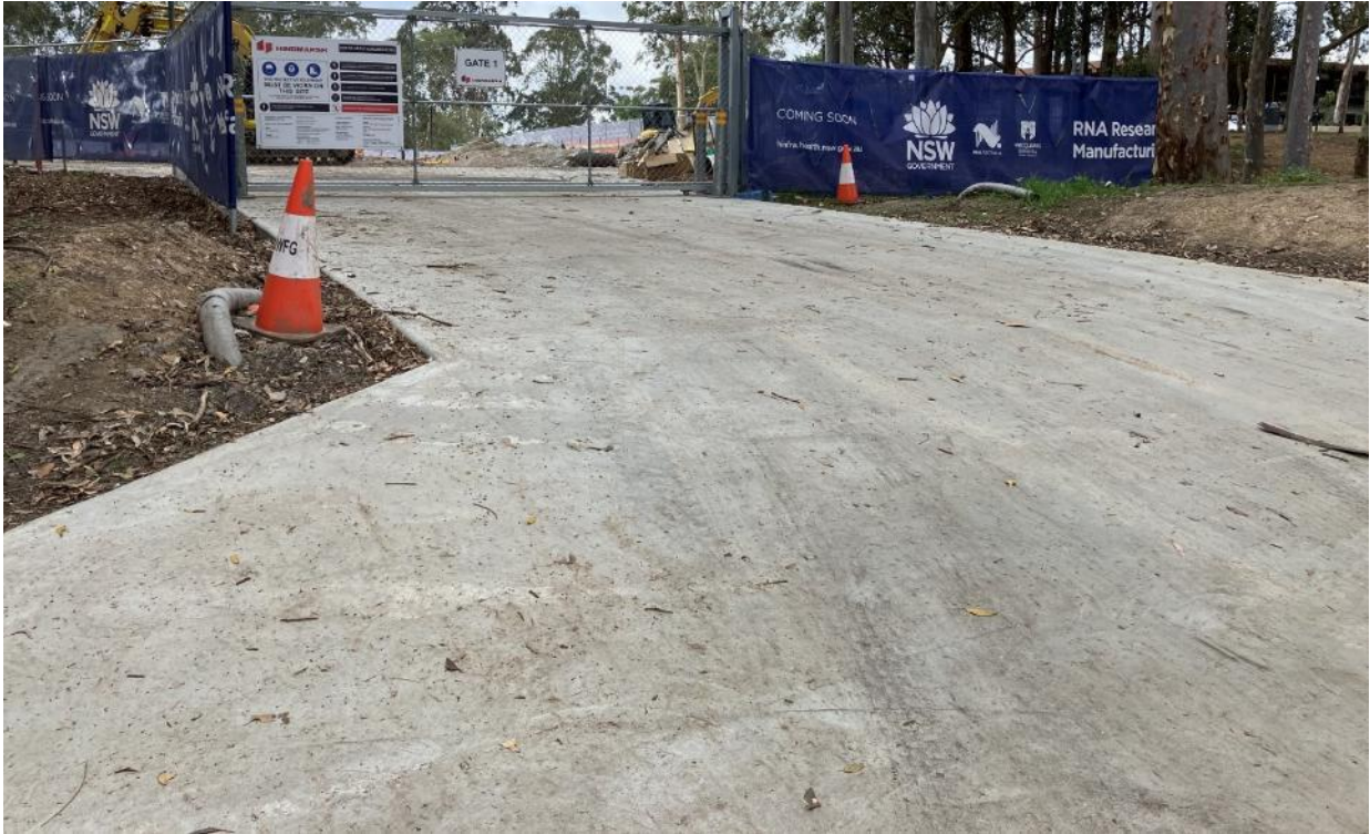
OBS-04: Some minor tracking from site access driveway observed at Gate 1.
