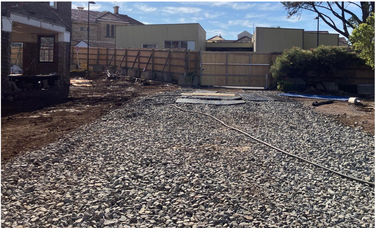
Rocks placed for stabilisation at Chatterry site. Access gate leads to Cleaners Building.
