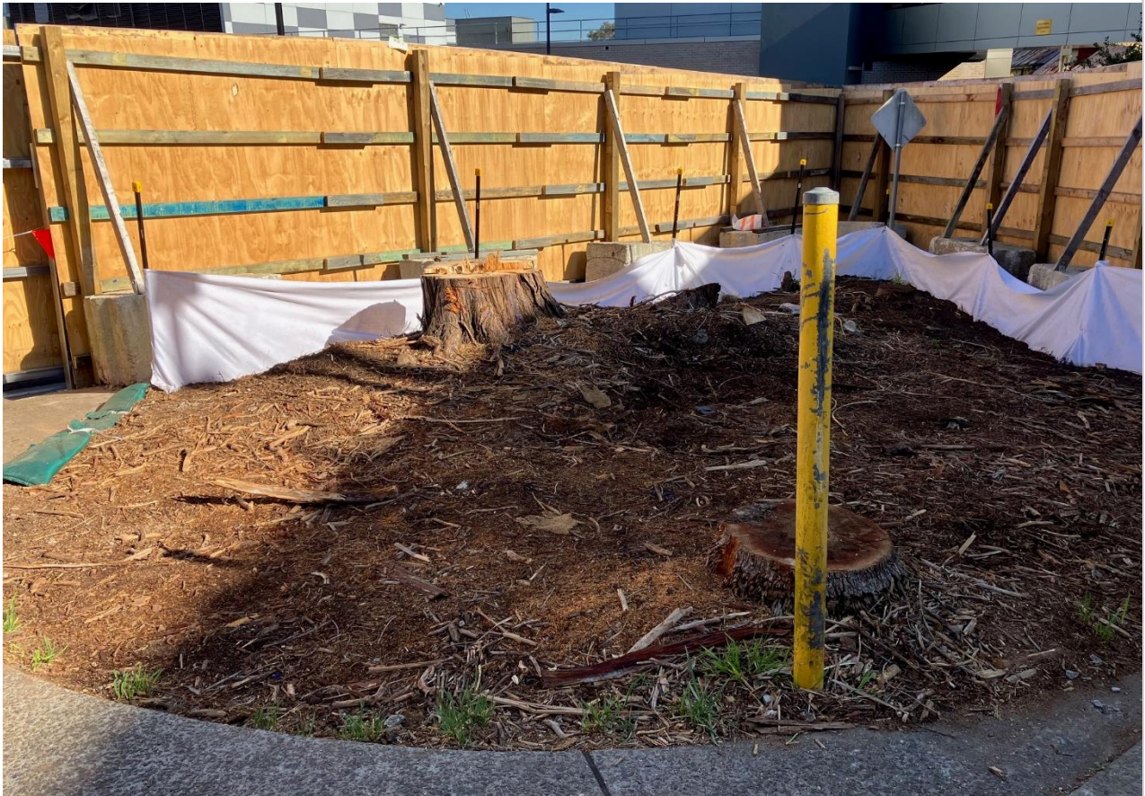
Cleaners Building site. Tree clearing complete with stumps to be removed following demolition.
