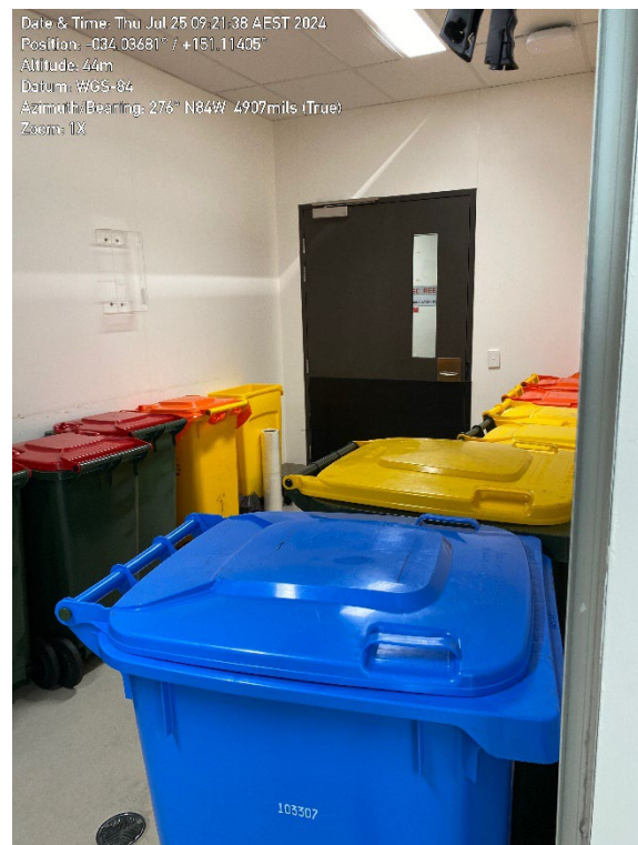
Internal waste storage room.
