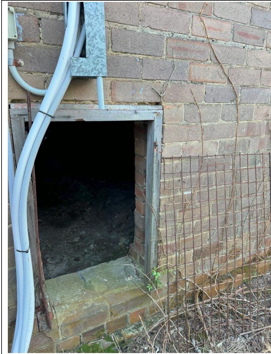
Plate 5: Example of an opening into the crawl space under the building inspected.
